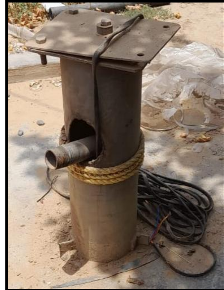
Installation of Submersible Pump at Govt. Primary School, Aasin ki Dhani, Dhiryawas
