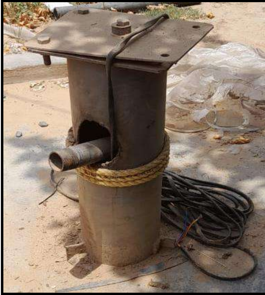
Installation of Submersible Pump at Govt. Primary School, Aasin ki Dhani, Dhiryawas
